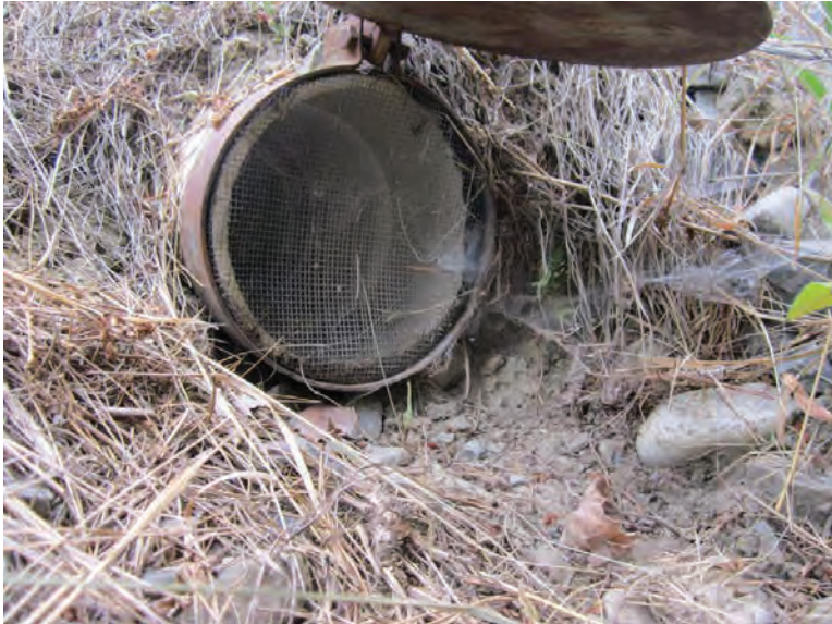
Photograph 35: Parker Canyon tank screened overflow w metal flapper valve
