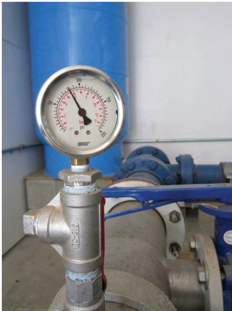
Photograph 46: Four Corners inlet pressure
