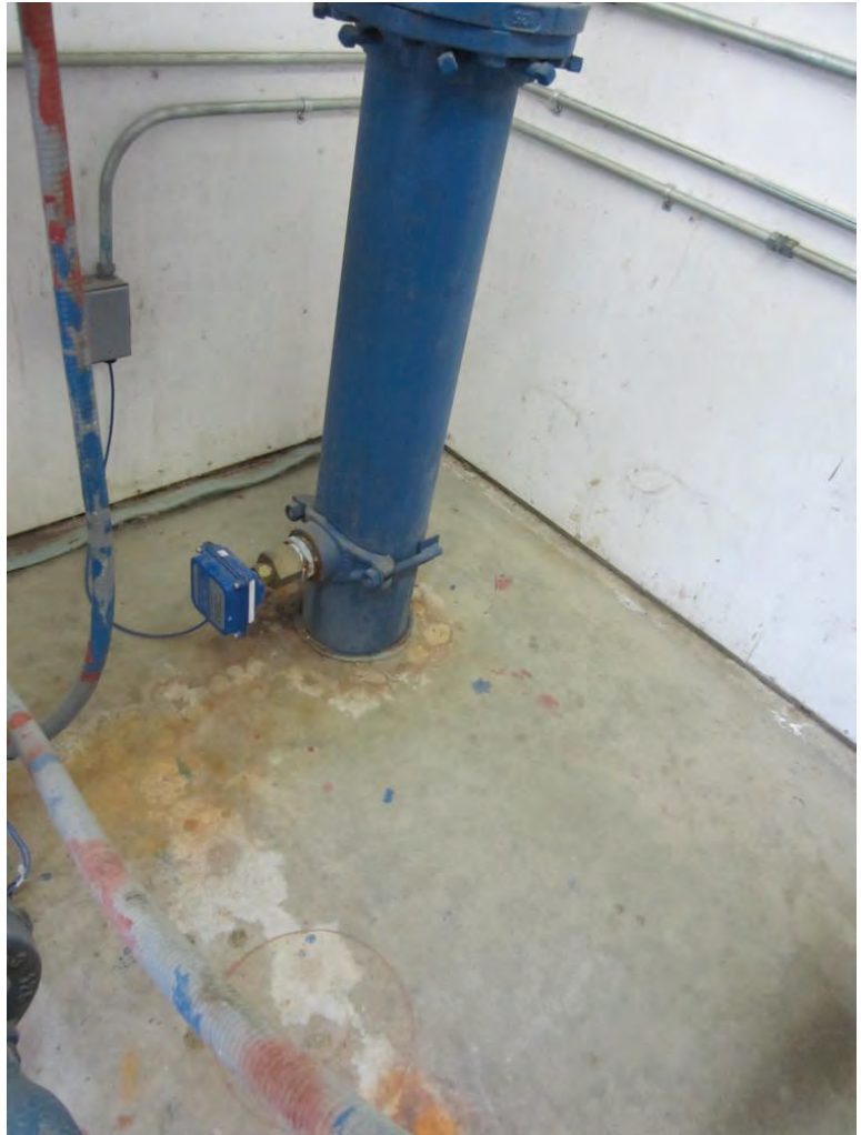
Photograph 94: Highland Flats combined boosted discharge flow meter
