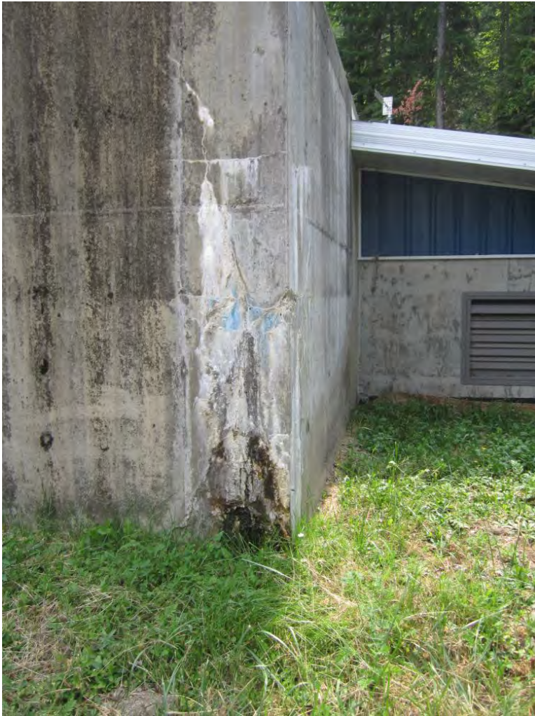
Photograph 49: Black Mountain reservoir (leak)
