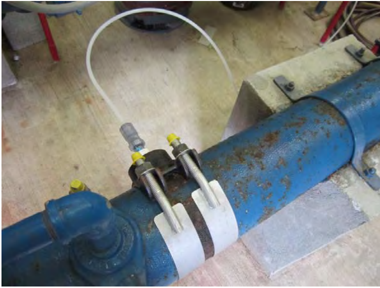
Photograph 13: Sodium hypochlorite injection quill
