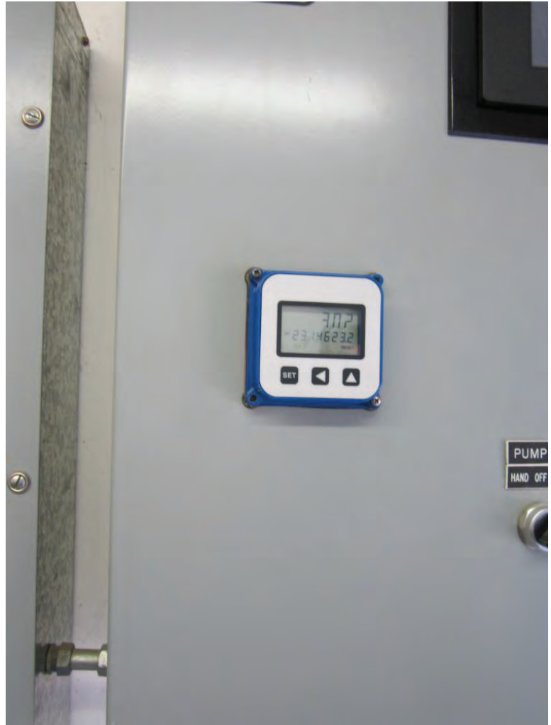
Photograph 92: Highland Flats flow meter (malfunctioning)
