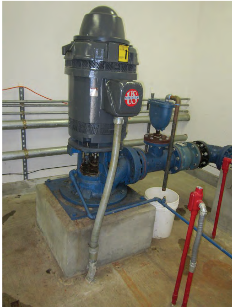
Photograph 30: Parker Canyon booster pump
