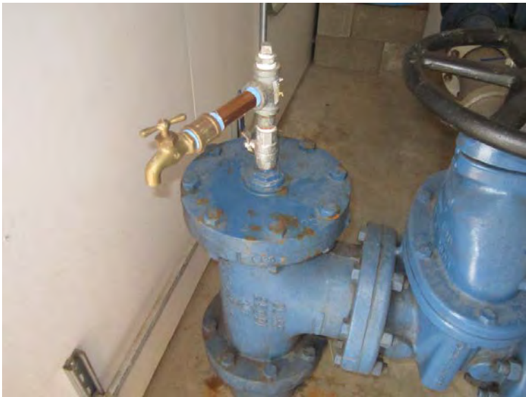
Photograph 43: Four Corners sample tap
