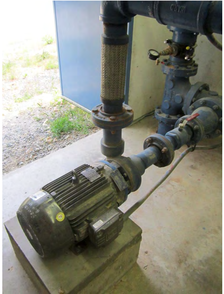
Photograph 98: Highland Flats booster pump
