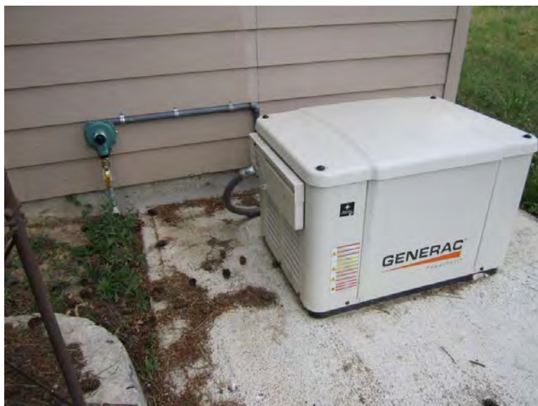
Photograph 48: Four Corners propane generator
