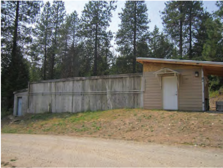
Photograph 73: Naples tank and booster station
