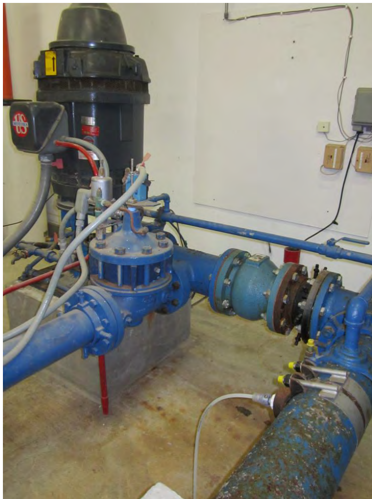
Photograph 18: Well 2 discharge to waste control valve
