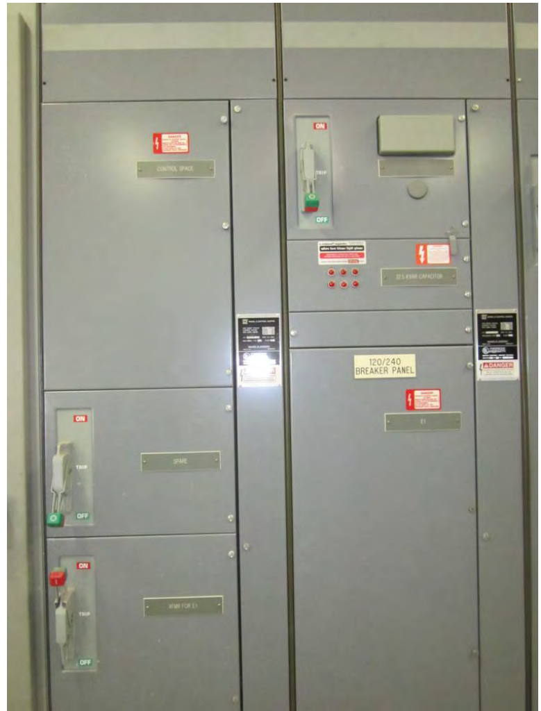
Photograph 20: Well electrical switches
