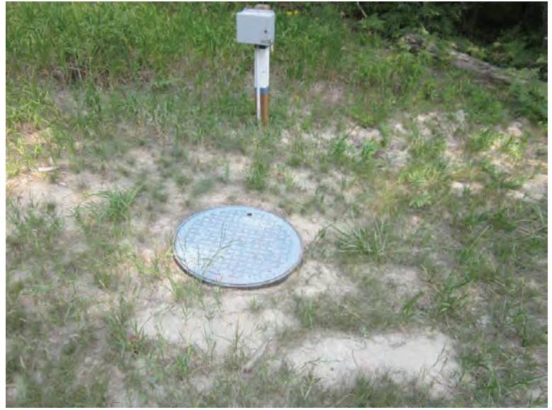
Photograph 70: Pressure reducing valve vault w pigtail
