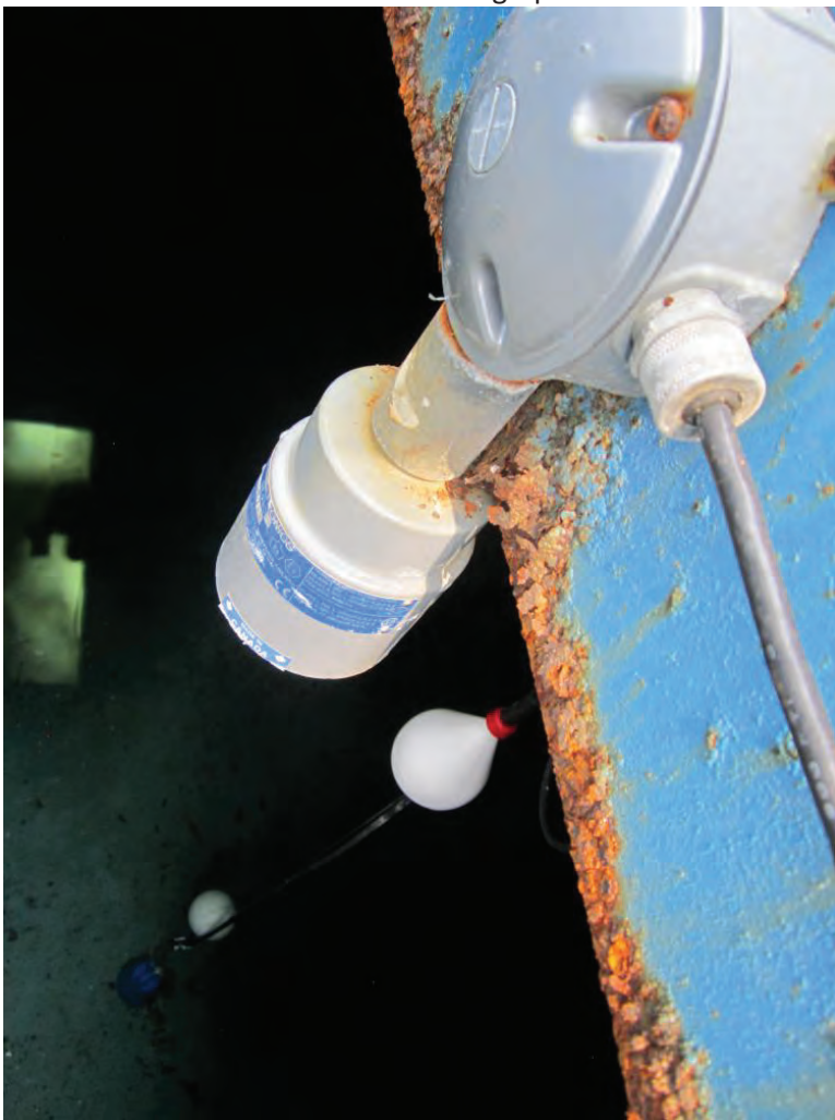
Photograph 83: Naples tank ultra-sonic level transducer
