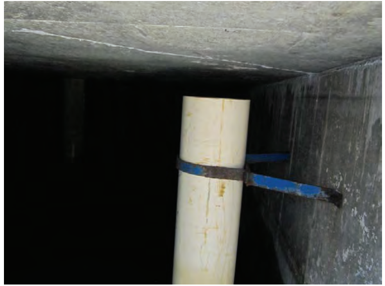
Photograph 54: Black Mountain reservoir interior overflow
