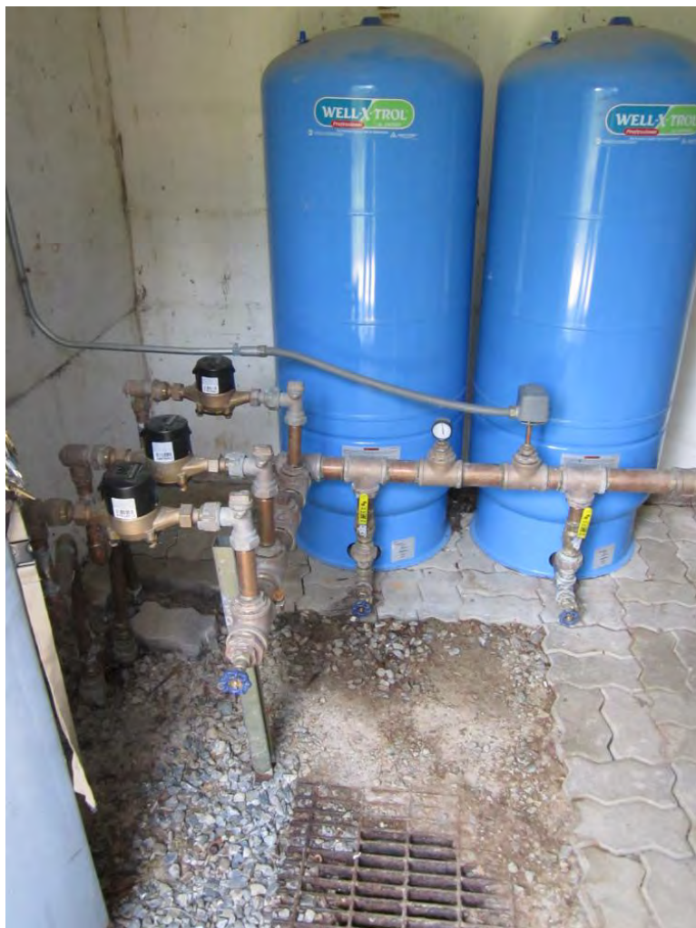
Photograph 76: Naples tank booster station, 3 residential connections
