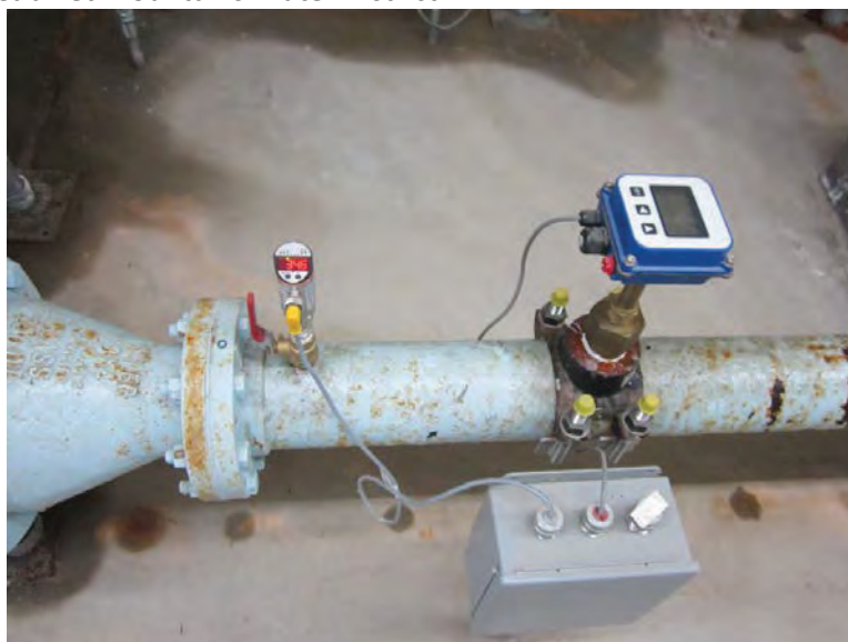
Photograph 62: Black Mountain boosted discharge flow meter
