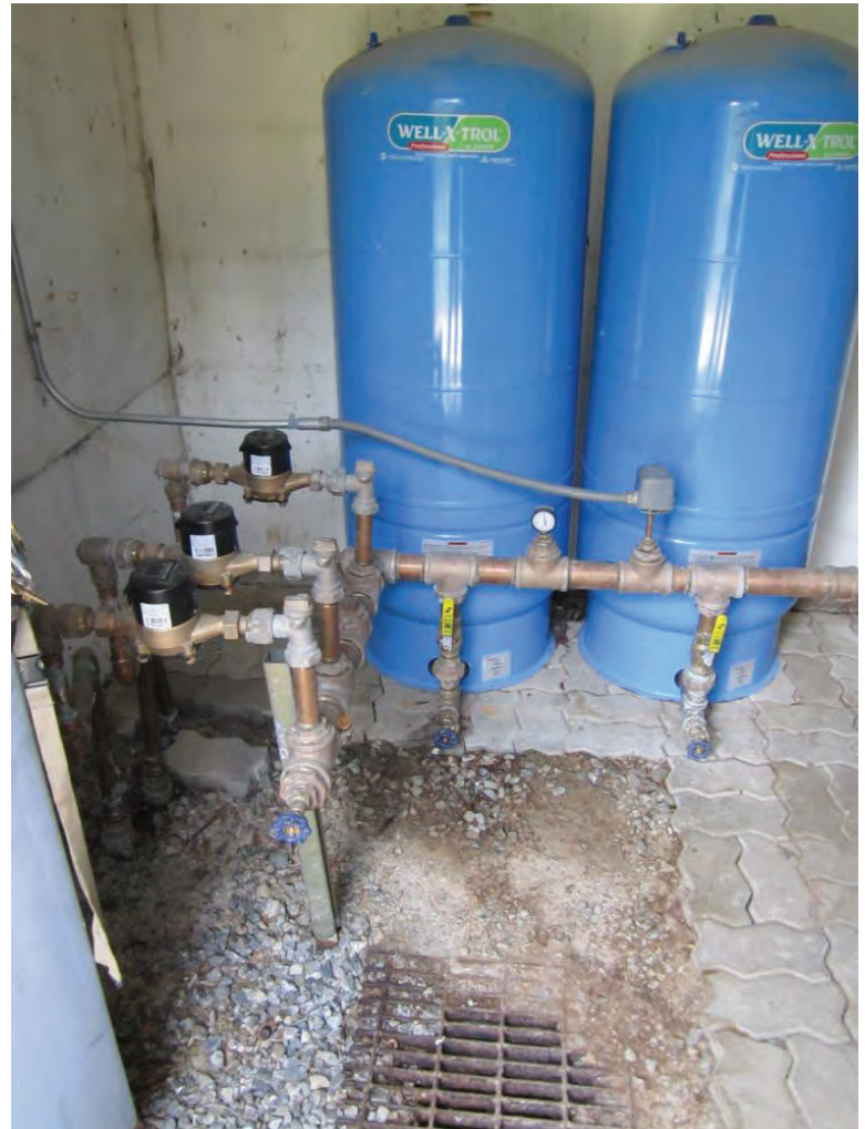
Photograph 76: Naples tank booster station, 3 residential connections
