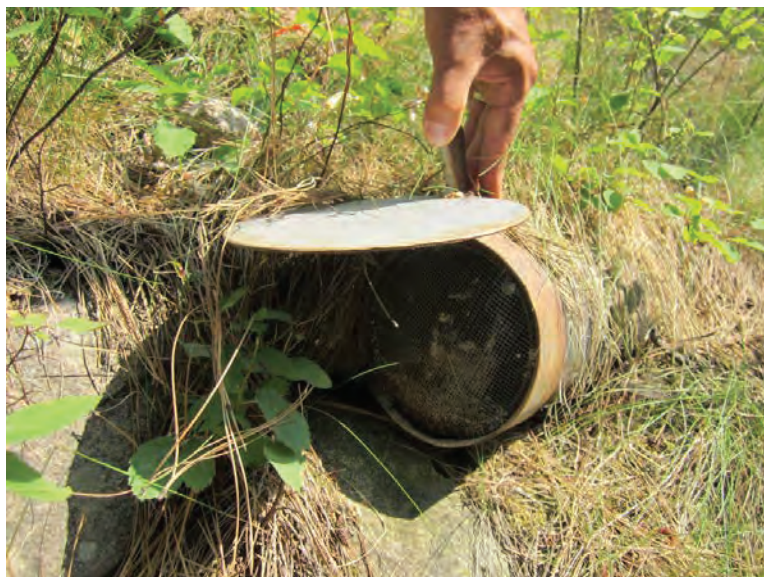
Photograph 80: Naples tank overflow outlet screened with metal flapper valve
