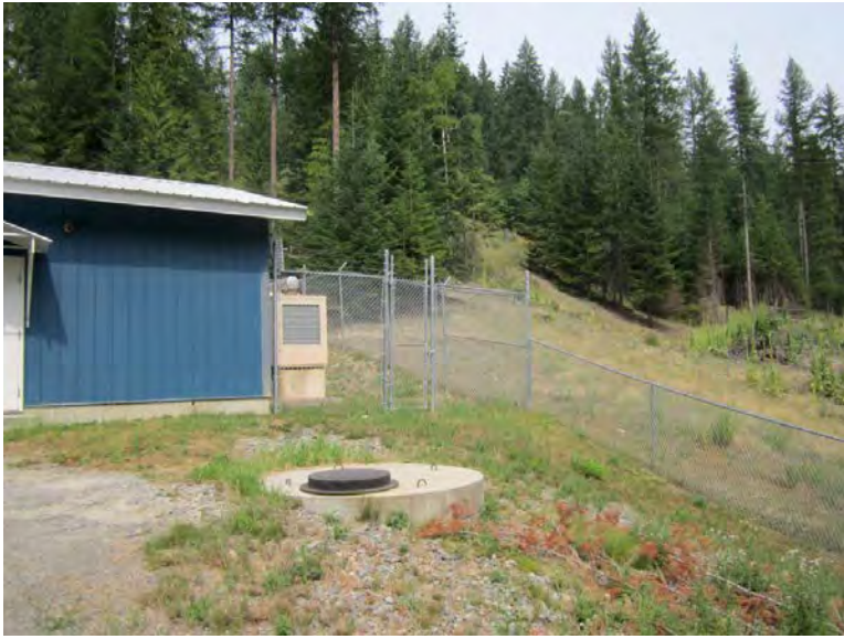
Photograph 25: Parker Canyon diesel generator
