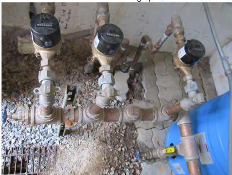
Photograph 77: Naples tank boosted discharge, 3 residential connections
