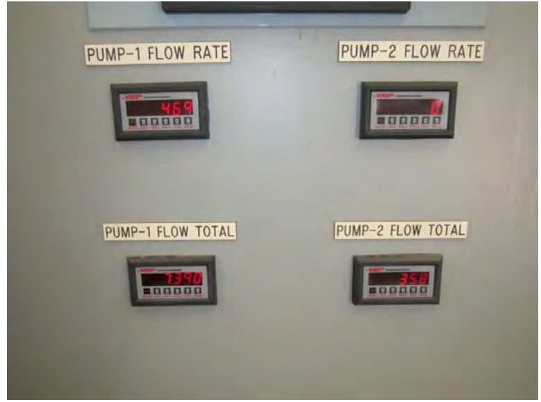
Photograph 34: Parker Canyon pump controls
