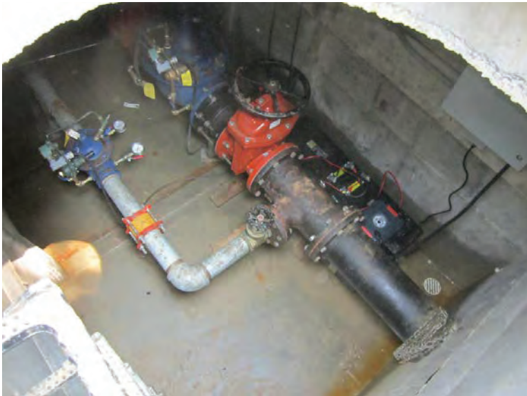
Photograph 71: Pressure reducing valve vault
