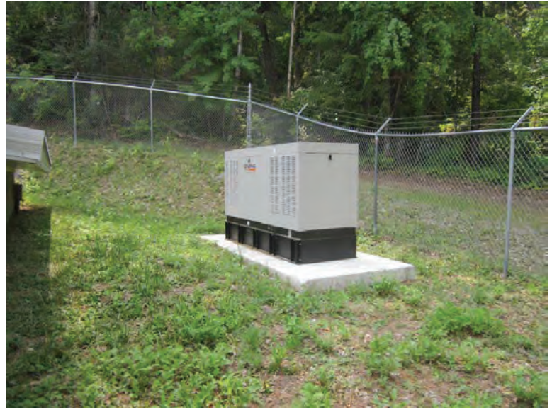
Photograph 58: Black Mountain booster station diesel generator
