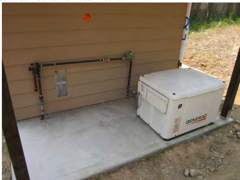
Photograph 74: Naples booster station propane generator
