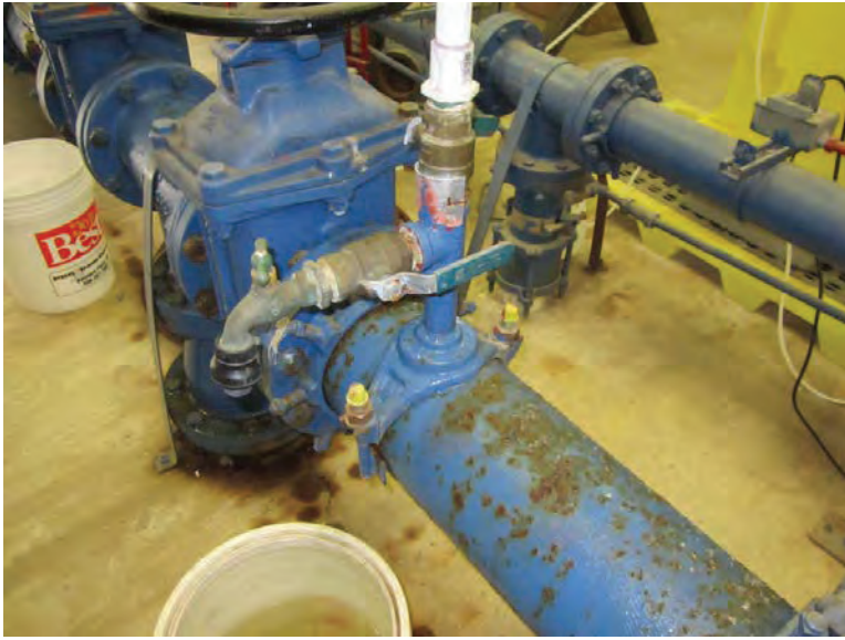
Photograph 17: Finished (chlorinated) sample tap
