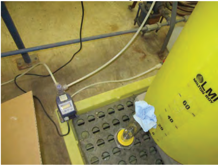
Photograph 9: Well 2 electronic metering pump and calibration cylinder
