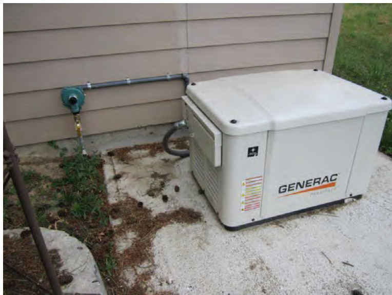
Photograph 48: Four Corners propane generator
