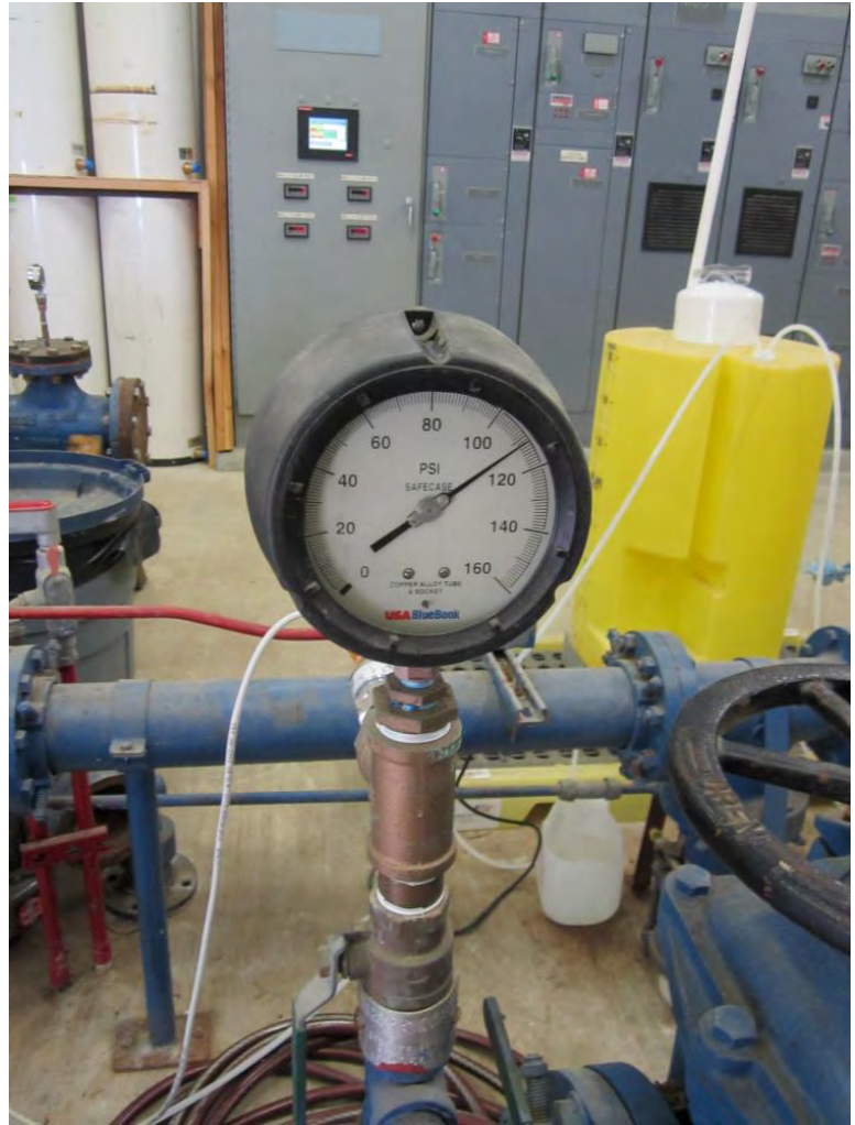
Photograph 14: Pressure gage well discharge
