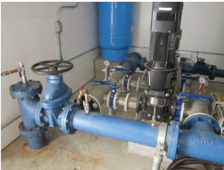
Photograph 39: Four Corners booster station
