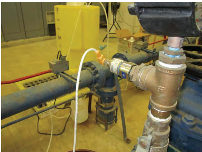
Photograph 15: Pressure transducer on combined well discharge
