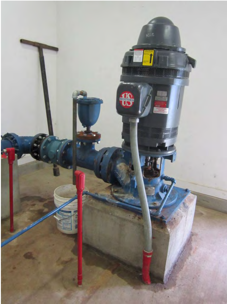
Photograph 29: Parker Canyon booster pump
