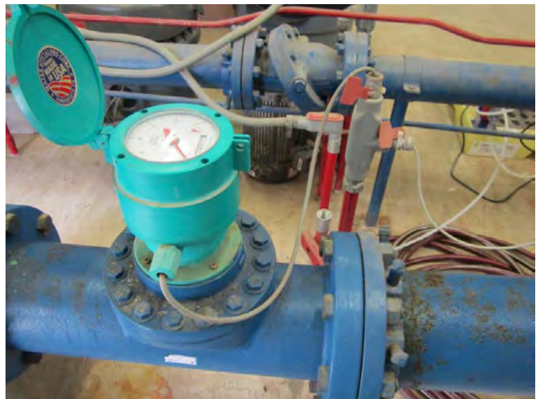
Photograph 16: Individual flow meter tied to electronic chlorine metering pump
