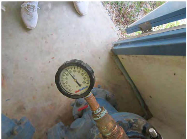
Photograph 96: Highland Flats inlet pressure
