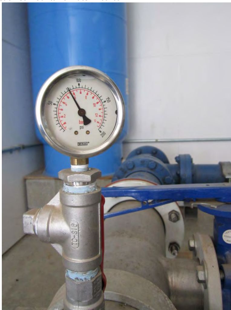
Photograph 46: Four Corners inlet pressure
