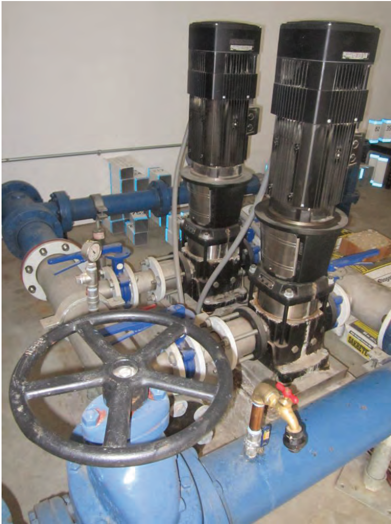
Photograph 41: Four Corners booster pumps and discharge appurtenances
