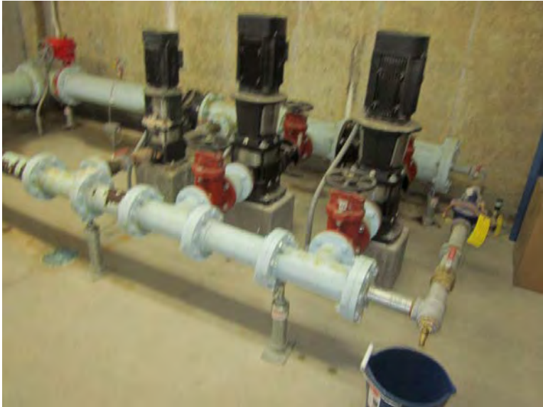
Photograph 59: Black Mountain booster pumps and discharge appurtenances
