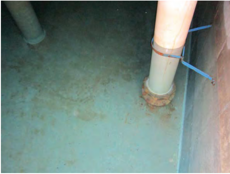
Photograph 53: Black Mountain reservoir interior overflow
