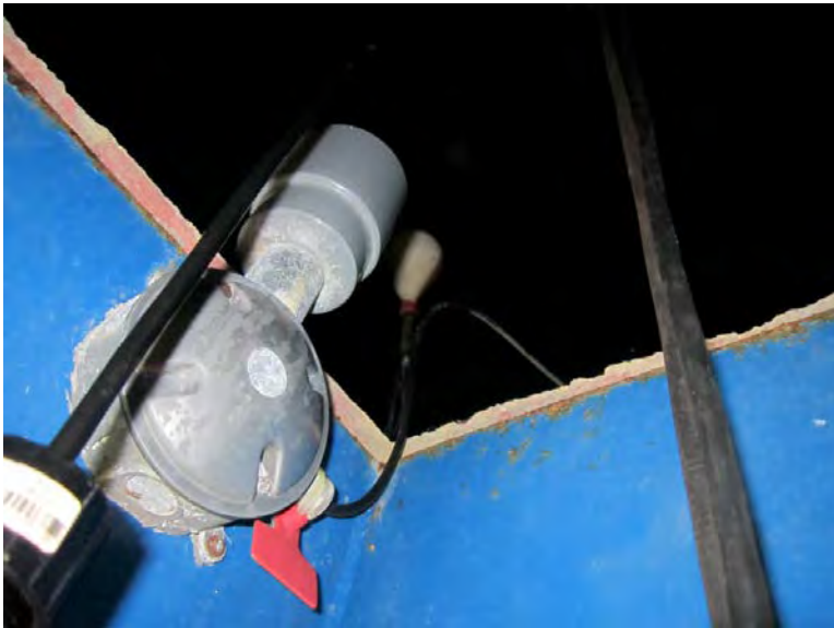
Photograph 27: Parker Canyon level controls (well actuation)
