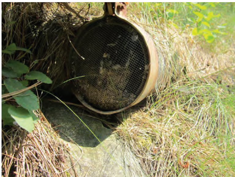
Photograph 79: Naples tank overflow outlet screened with metal flapper valve
