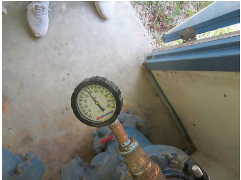
Photograph 96: Highland Flats inlet pressure
