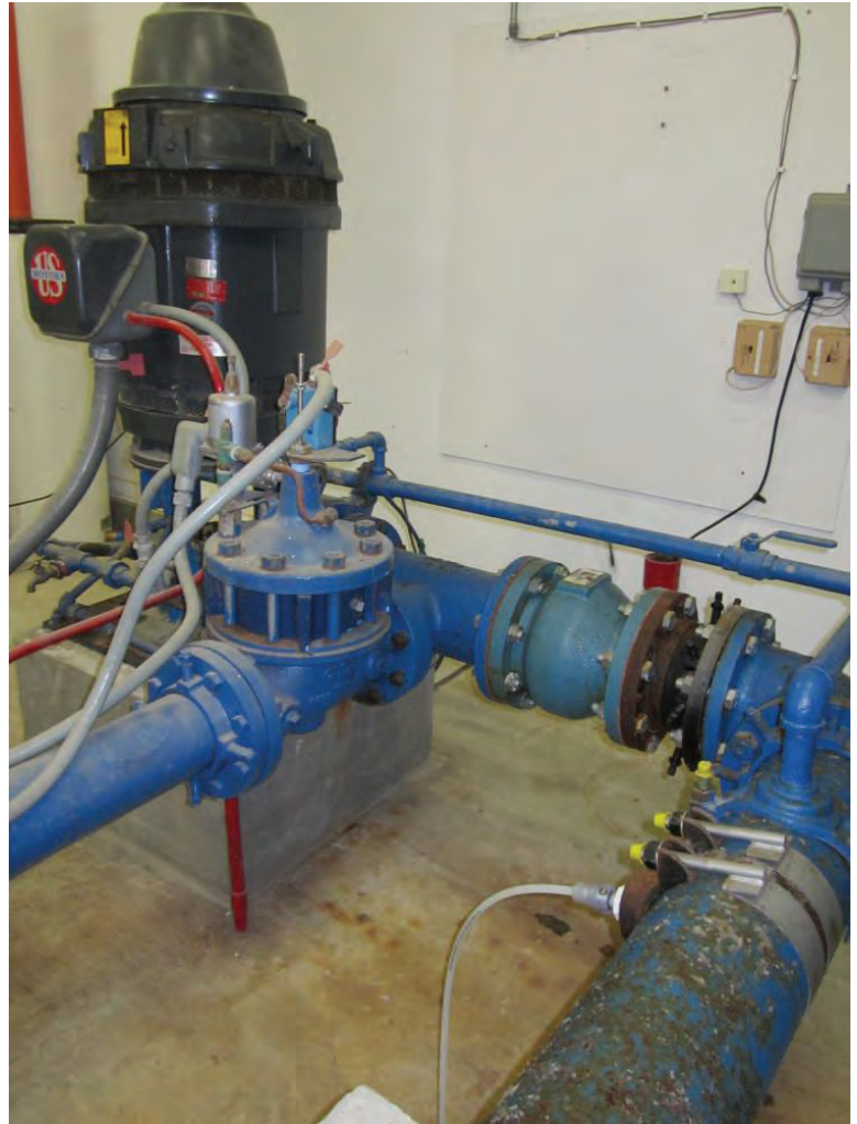
Photograph 18: Well 2 discharge to waste control valve
