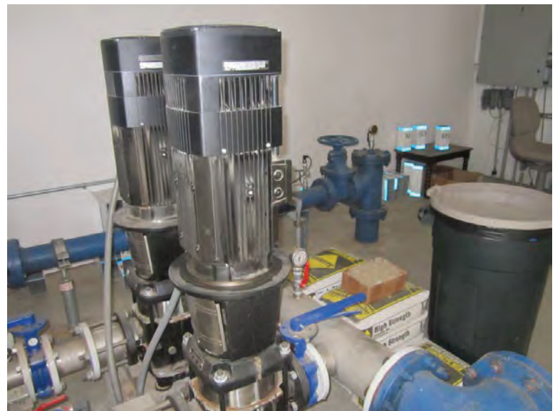
Photograph 40: Four Corners booster pumps and discharge appurtenances
