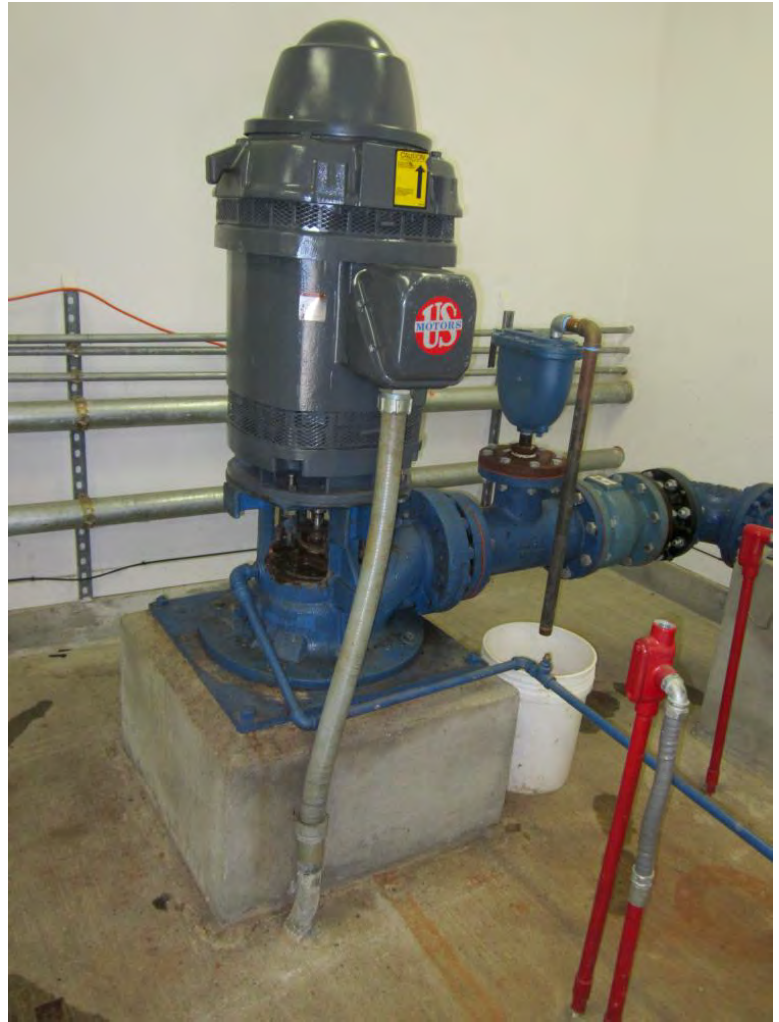
Photograph 30: Parker Canyon booster pump
