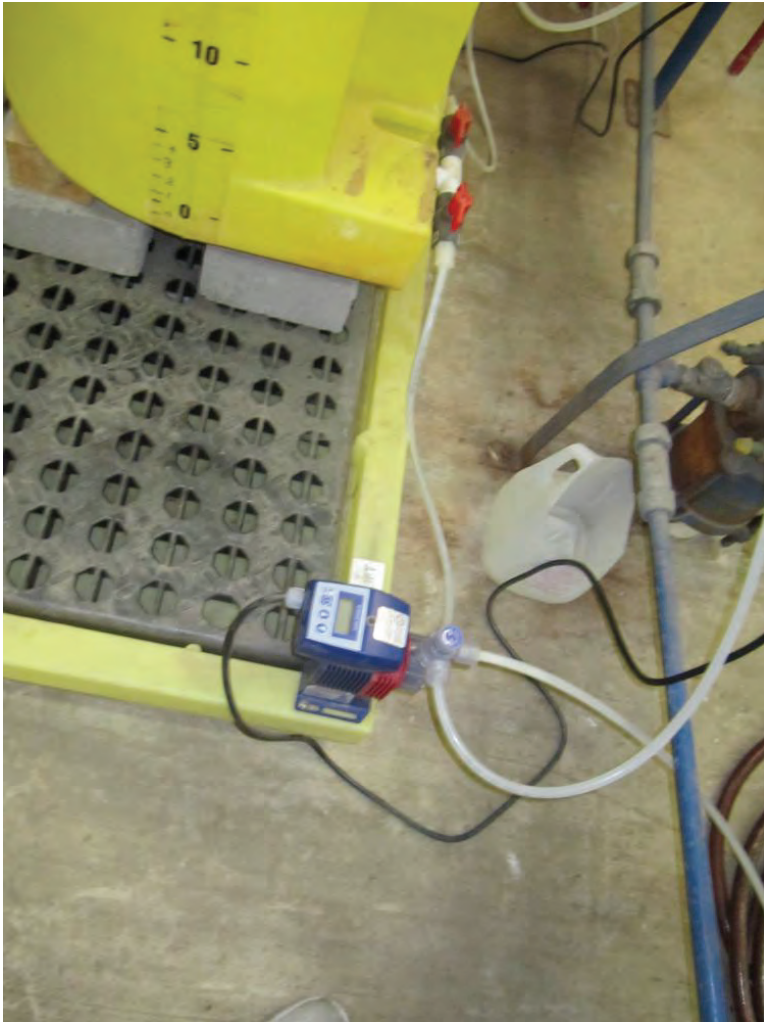
Photograph 11: Well 1 electronic metering pump
