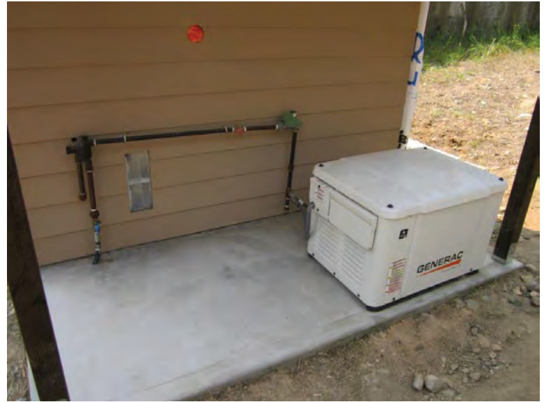
Photograph 74: Naples booster station propane generator
