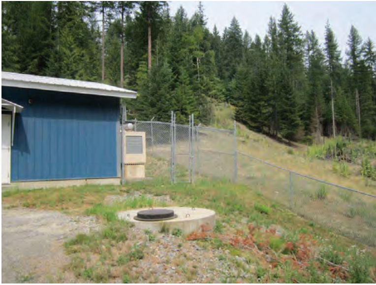
Photograph 25: Parker Canyon diesel generator
