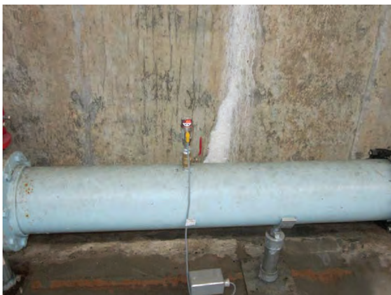
Photograph 63: Black Mountain boosted discharge appurtenances flow meter
