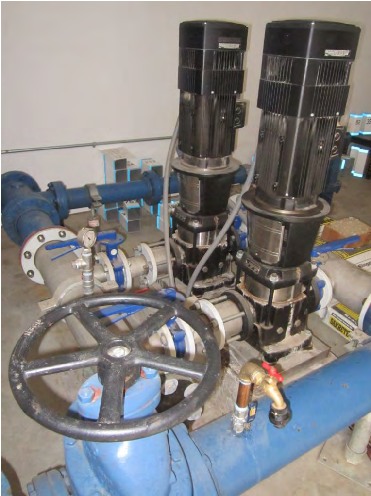
Photograph 41: Four Corners booster pumps and discharge appurtenances
