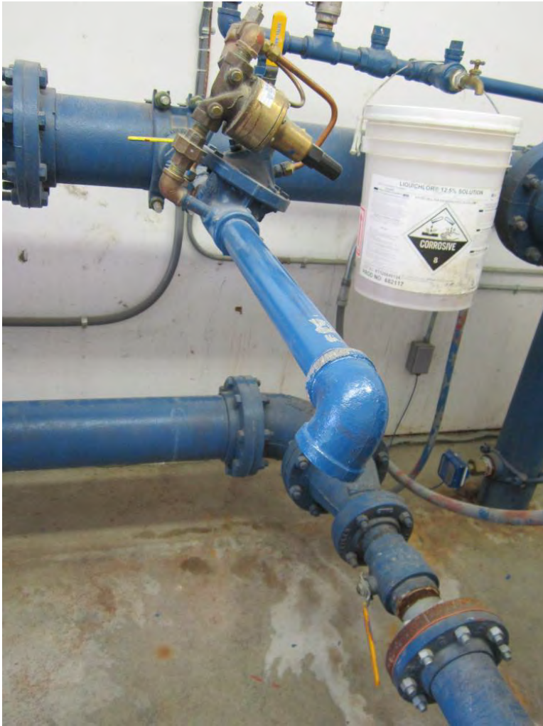
Photograph 93: Highland Flats pressure relief (requires reconfiguration of discharge)
