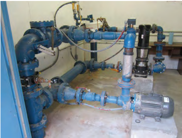
Photograph 95: Highland Flats boosted discharge appurtenances
