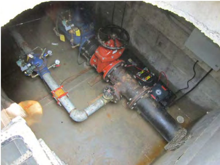
Photograph 71: Pressure reducing valve vault
