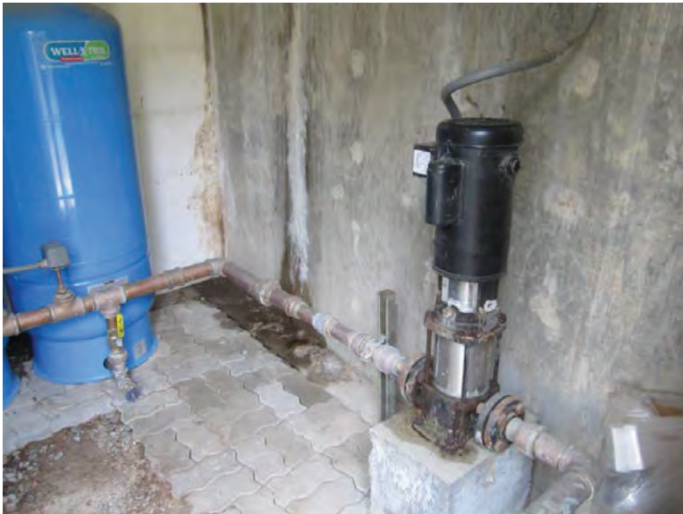
Photograph 75: Naples tank booster pump
