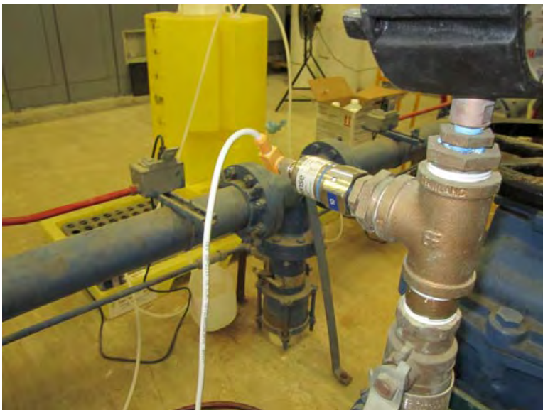
Photograph 15: Pressure transducer on combined well discharge
