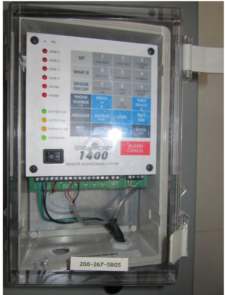
Photograph 38: Four Corners booster station autodialer
