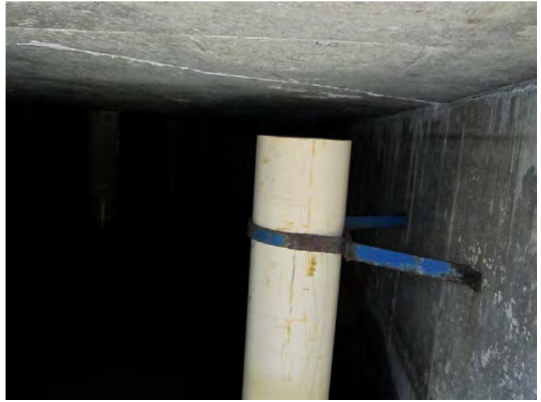
Photograph 54: Black Mountain reservoir interior overflow
