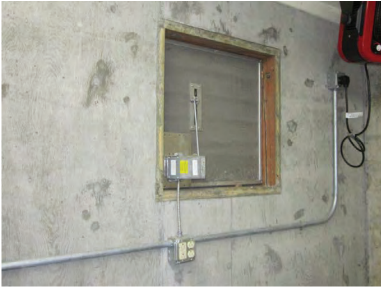
Photograph 65: Black Mountain booster station, thermostatically controlled louvre vent
