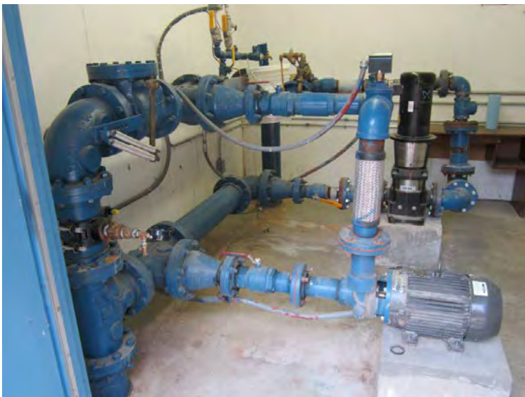
Photograph 95: Highland Flats boosted discharge appurtenances
