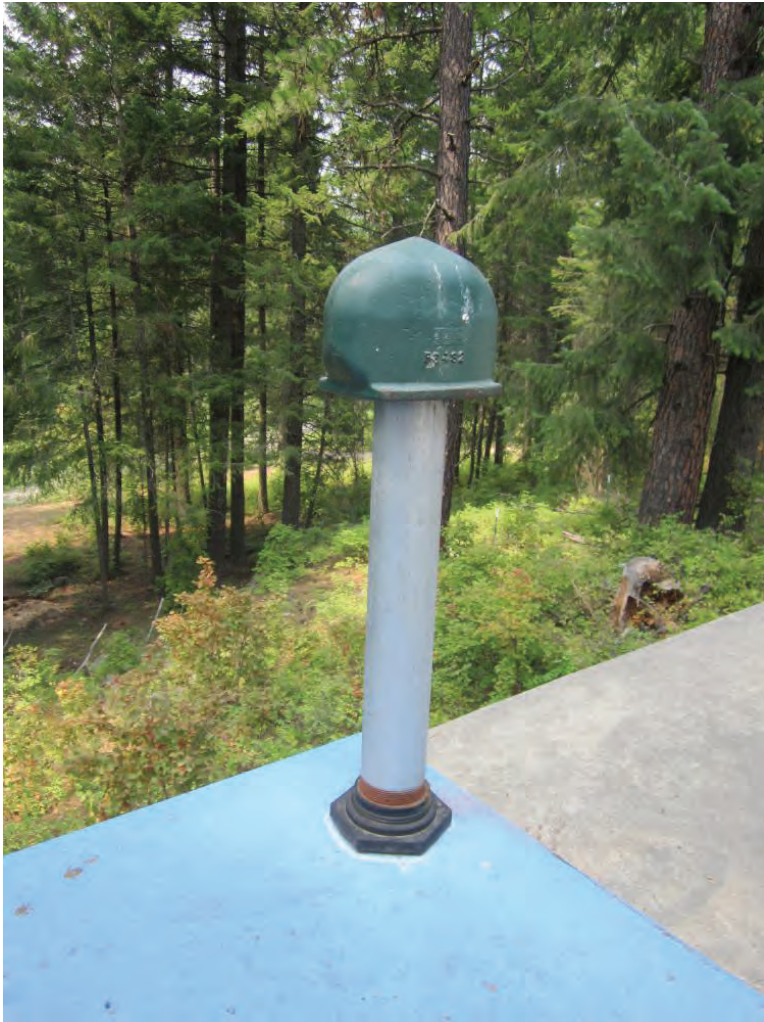
Photograph 87: Naples tank lid w screened vent
