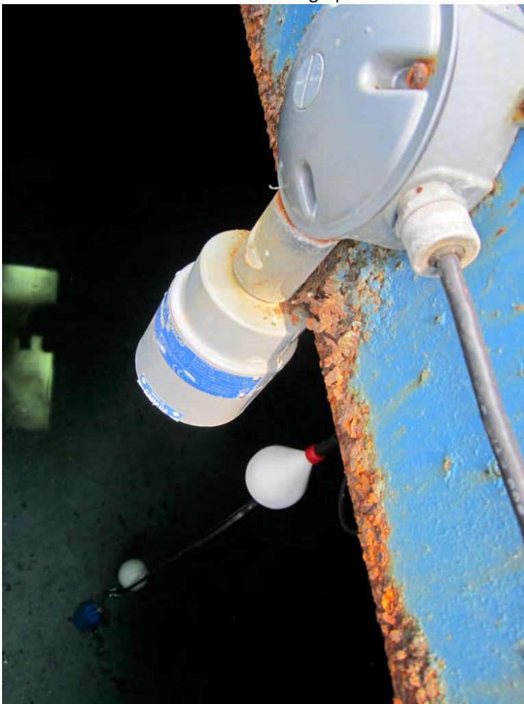
Photograph 83: Naples tank ultra-sonic level transducer
