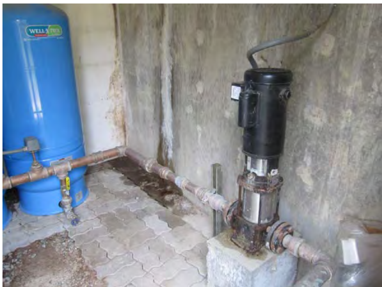
Photograph 75: Naples tank booster pump
