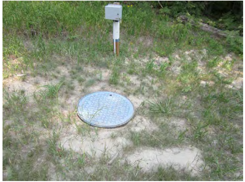
Photograph 70: Pressure reducing valve vault w pigtail
