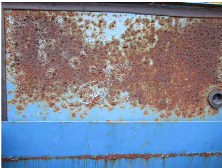
Photograph 86: Naples tank lid w water tight seal
