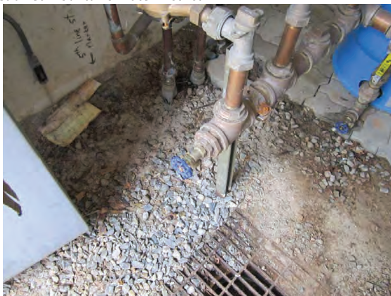
Photograph 78: Metered residential connection w corp stop
