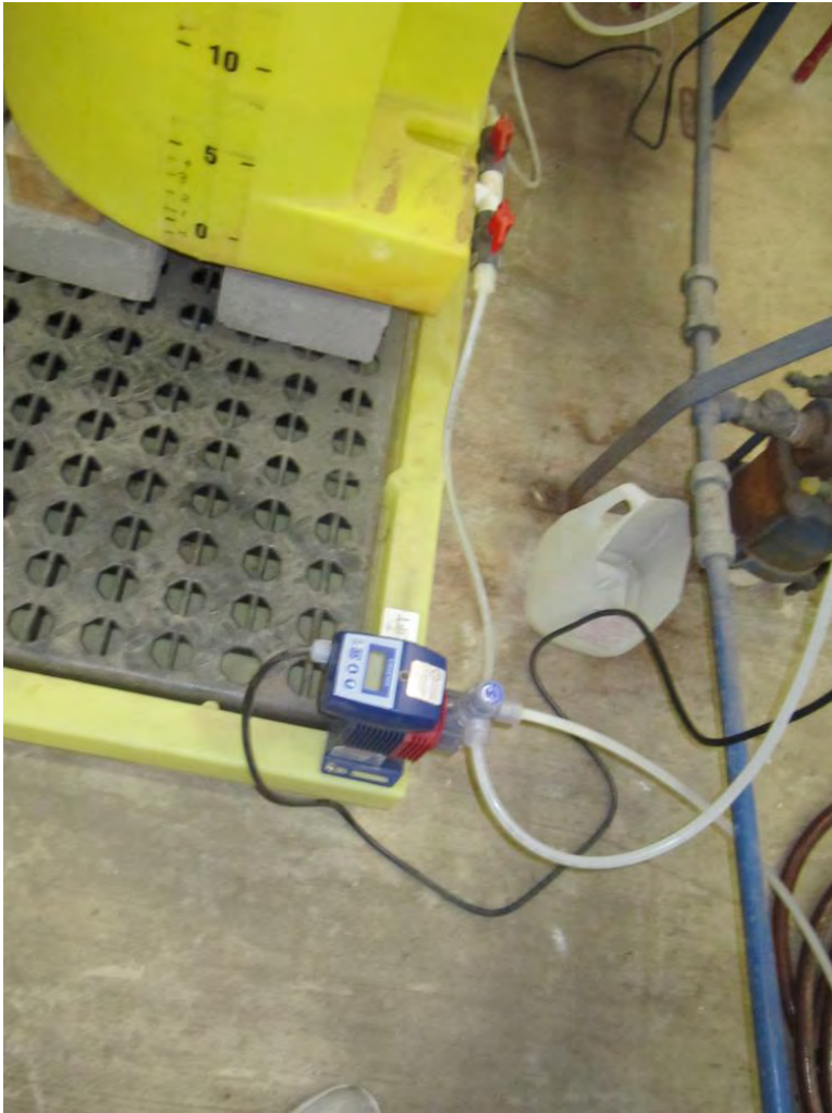
Photograph 11: Well 1 electronic metering pump
