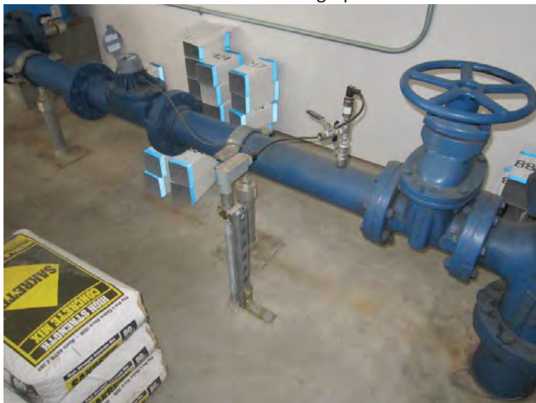
Photograph 45: Four Corners boosted discharge appurtenances
