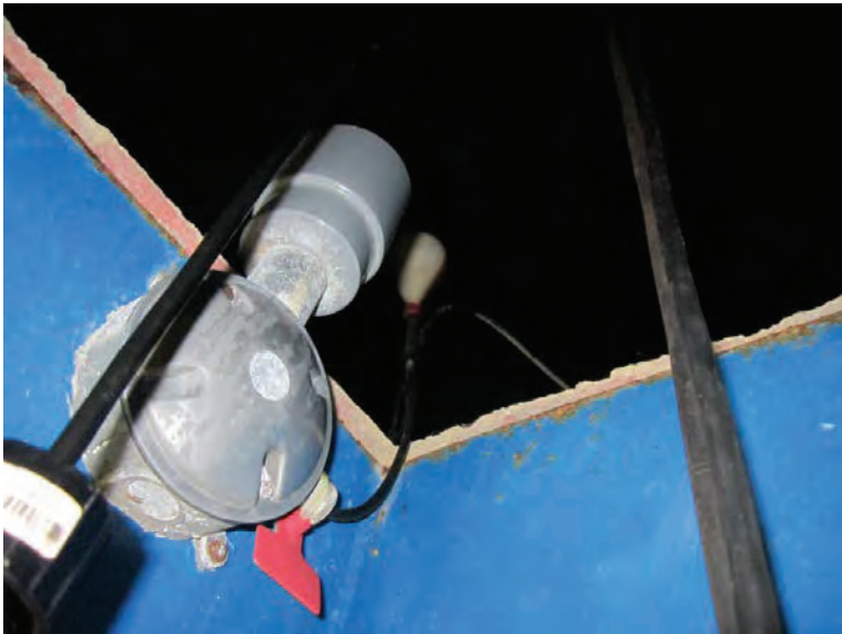
Photograph 27: Parker Canyon level controls (well actuation)
