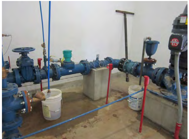
Photograph 32: Parker Canyon boosted discharge appurtenances
