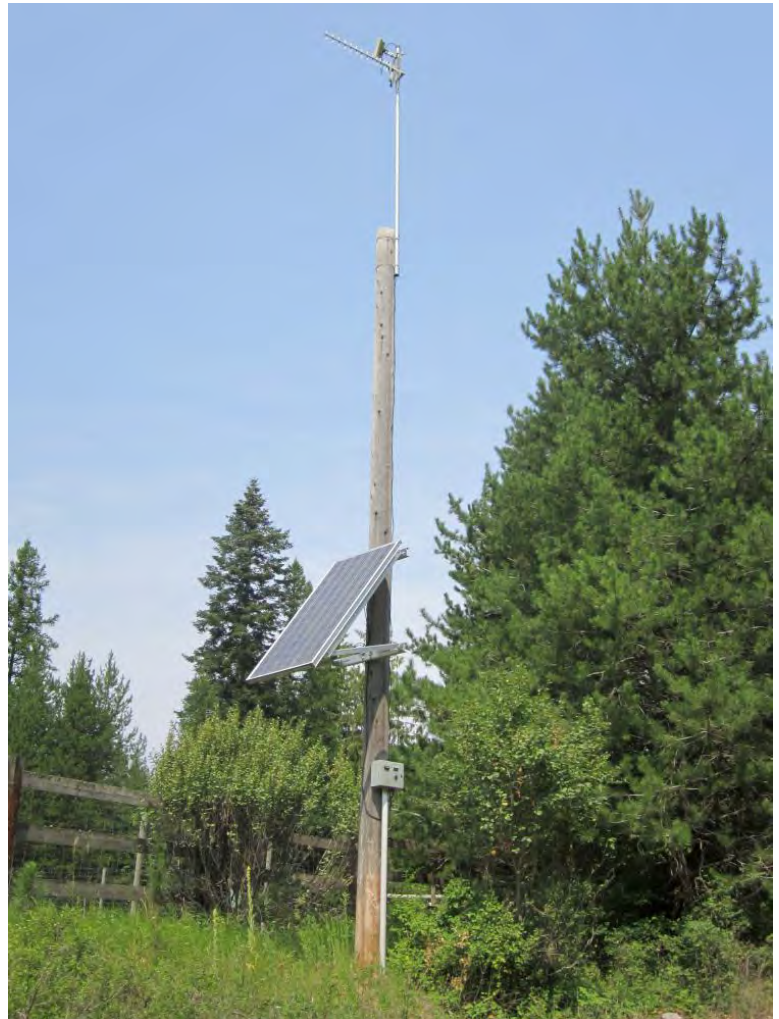
Photograph 72: Pressure reducing valve solar panel to charge batteries
