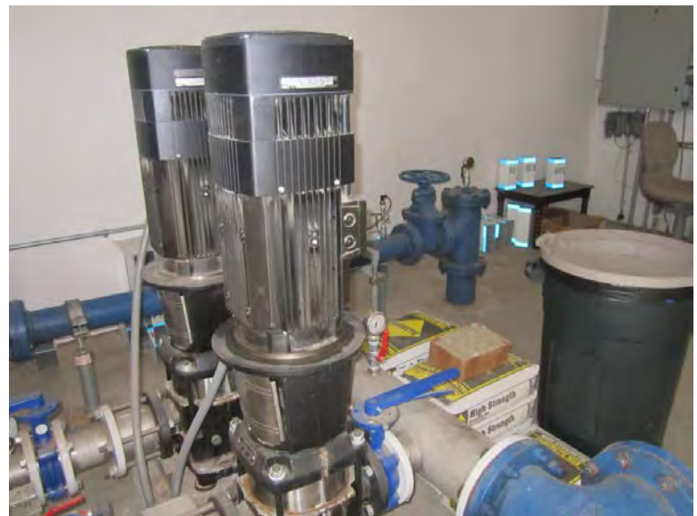
Photograph 40: Four Corners booster pumps and discharge appurtenances
