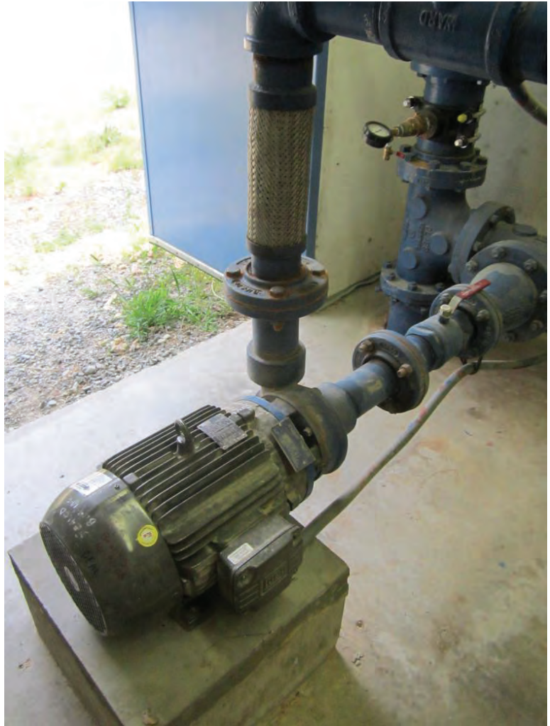
Photograph 98: Highland Flats booster pump
