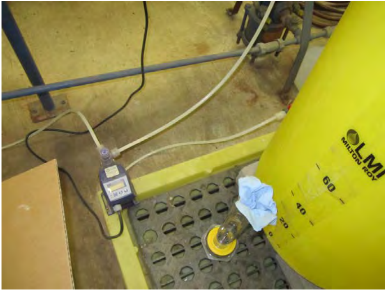
Photograph 9: Well 2 electronic metering pump and calibration cylinder
