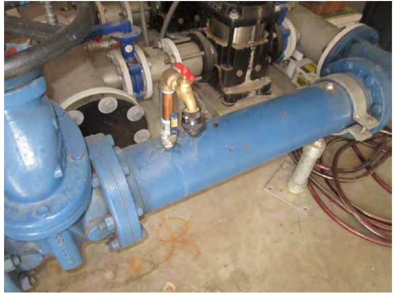
Photograph 42: Four Corners sample tap
