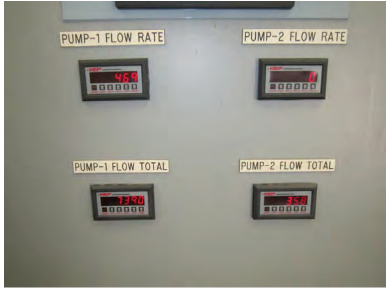
Photograph 34: Parker Canyon pump controls
