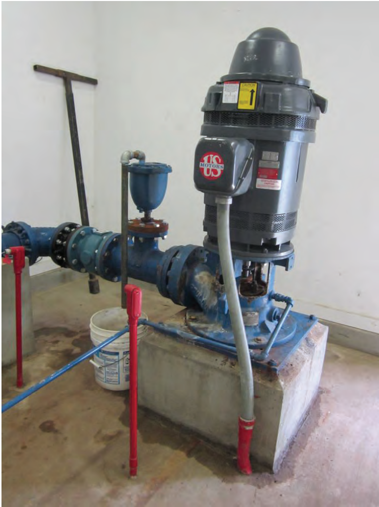
Photograph 29: Parker Canyon booster pump
