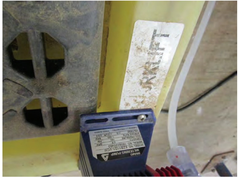
Photograph 12: Electronic metering pump placard
