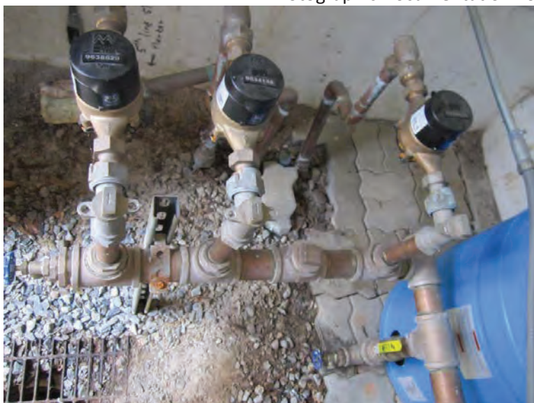
Photograph 77: Naples tank boosted discharge, 3 residential connections
