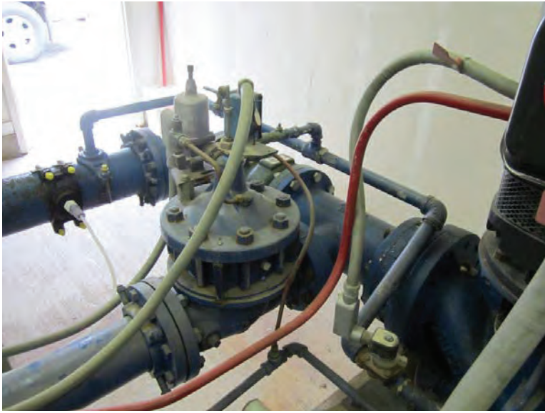
Photograph 5: Well 1 discharge to waste control valve
