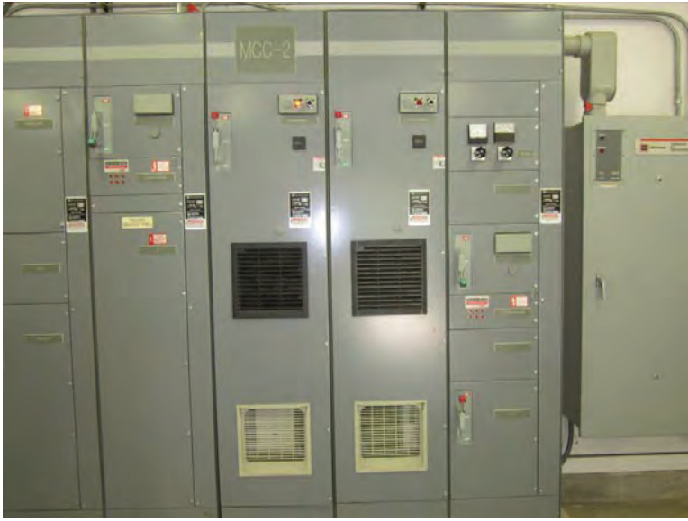
Photograph 33: Parker Canyon booster pump controls
