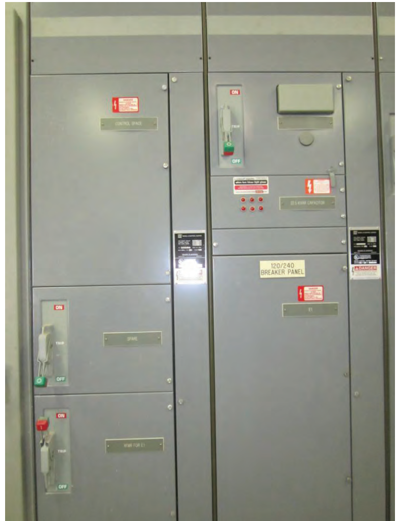
Photograph 20: Well electrical switches
