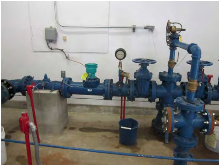
Photograph 31: Parker Canyon boosted discharge appurtenances
