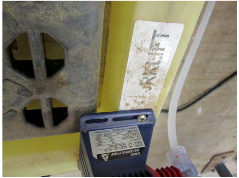
Photograph 12: Electronic metering pump placard
