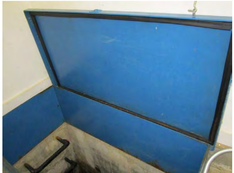
Photograph 28: Parker Canyon tank water tight access hatch
