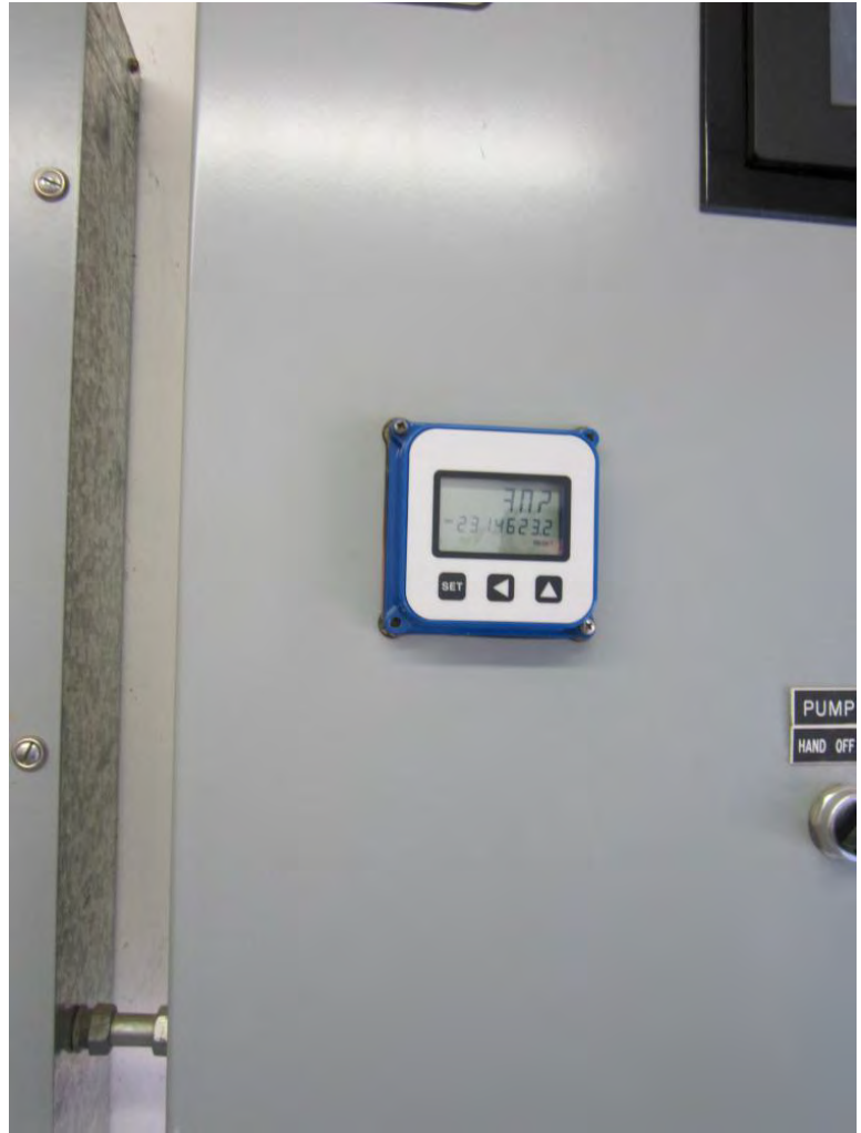
Photograph 92: Highland Flats flow meter (malfunctioning)
