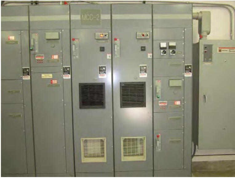
Photograph 33: Parker Canyon booster pump controls
