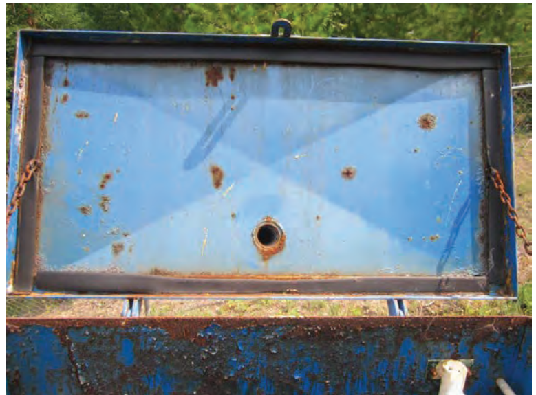
Photograph 52: Black Mountain interior reservoir hatch water tight seal
