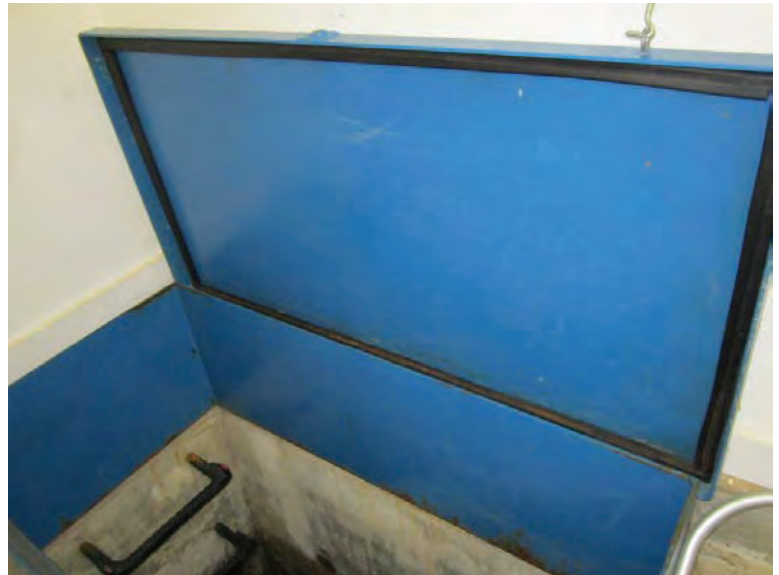
Photograph 28: Parker Canyon tank water tight access hatch
