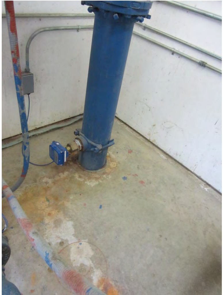
Photograph 94: Highland Flats combined boosted discharge flow meter
