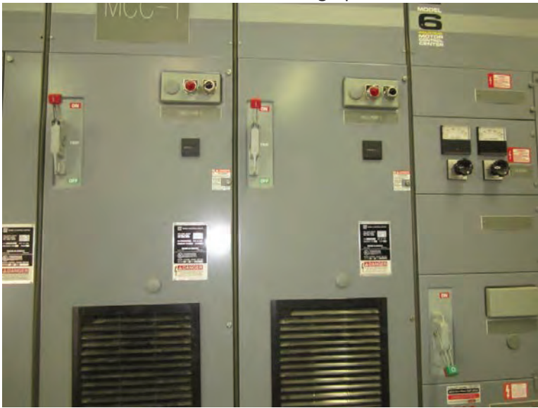
Photograph 19: Well electrical switches
