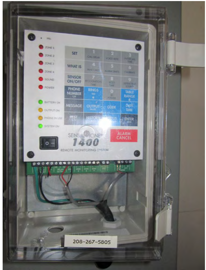
Photograph 38: Four Corners booster station autodialer
