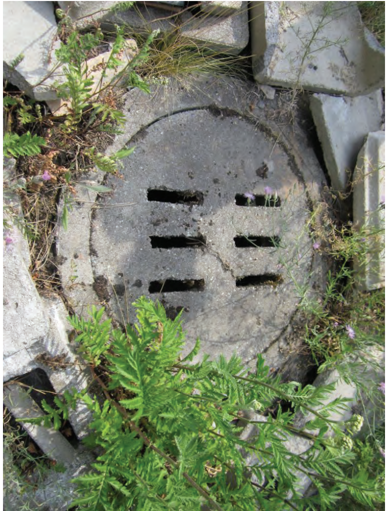
Photograph 22: Well discharge to waste dry well (requires air gap/backflow protection)
