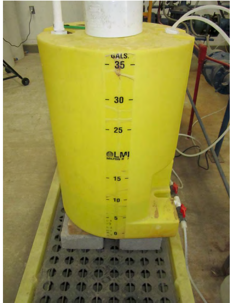
Photograph 10: Sodium hypochlorite day tank
