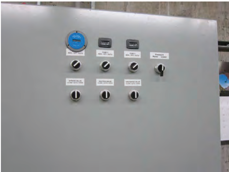
Photograph 67: Black Mountain booster pump controls
