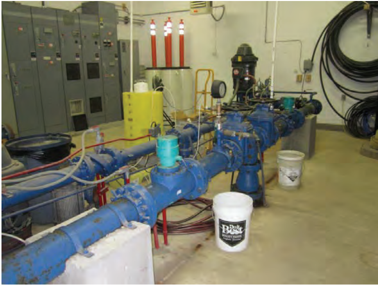
Photograph 1: Well discharge appurtenances
