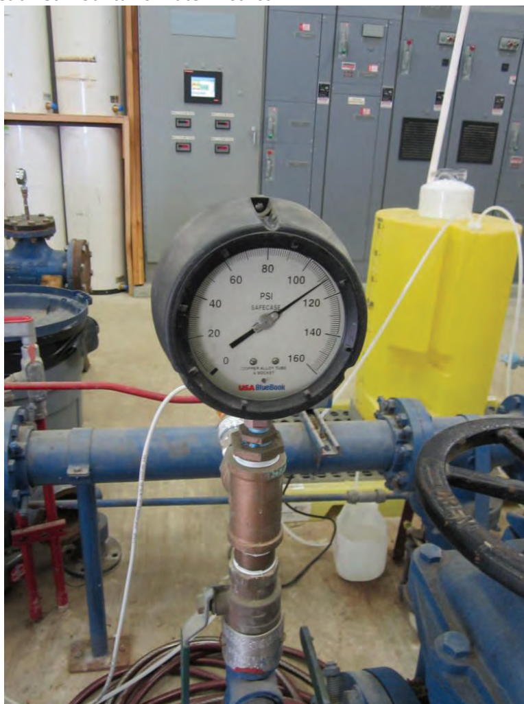
Photograph 14: Pressure gage well discharge
