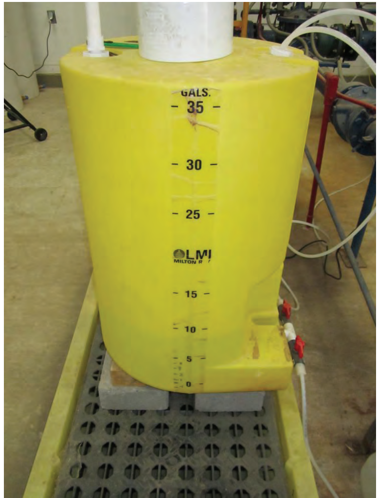
Photograph 10: Sodium hypochlorite day tank
