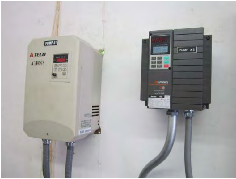
Photograph 91: Highland Flats booster pump controls
