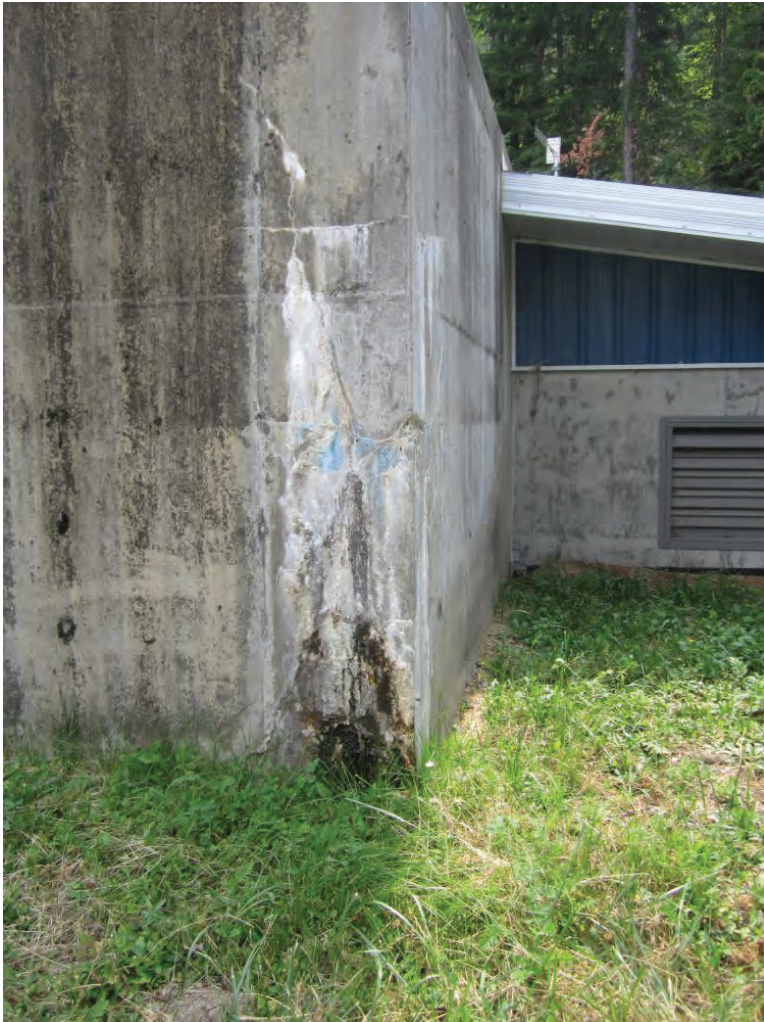
Photograph 49: Black Mountain reservoir (leak)
