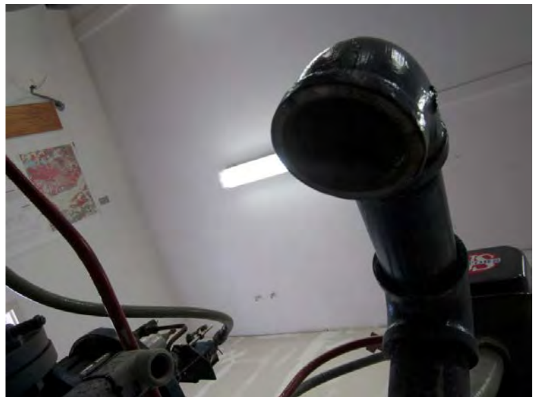
Photograph 4: Well 1 screened vent
