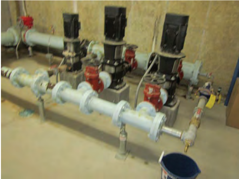
Photograph 59: Black Mountain booster pumps and discharge appurtenances
