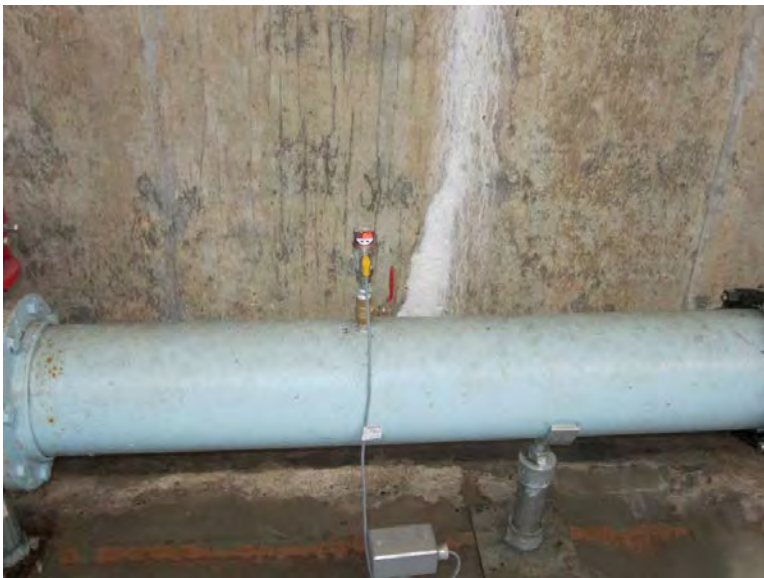
Photograph 63: Black Mountain boosted discharge appurtenances flow meter
