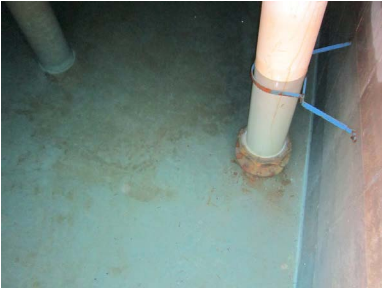
Photograph 53: Black Mountain reservoir interior overflow
