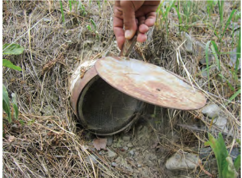
Photograph 36: Parker Canyon tank screened overflow w metal flapper valve
