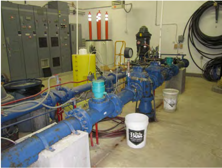
Photograph 1: Well discharge appurtenances
