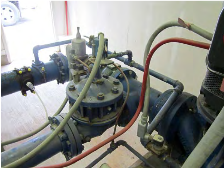
Photograph 5: Well 1 discharge to waste control valve
