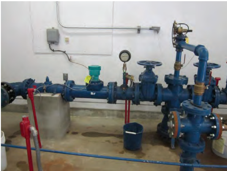
Photograph 31: Parker Canyon boosted discharge appurtenances
