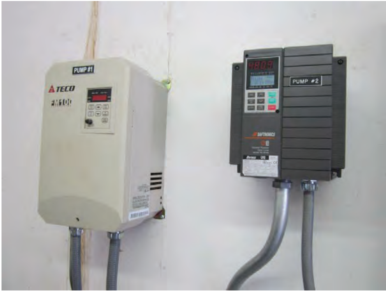
Photograph 91: Highland Flats booster pump controls
