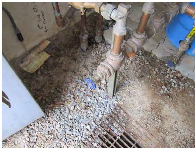
Photograph 78: Metered residential connection w corp stop
