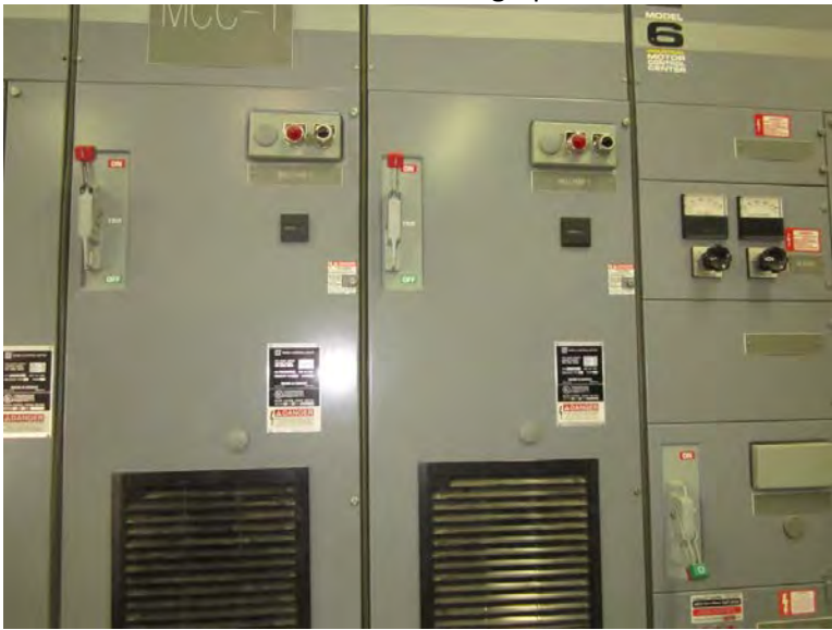
Photograph 19: Well electrical switches
