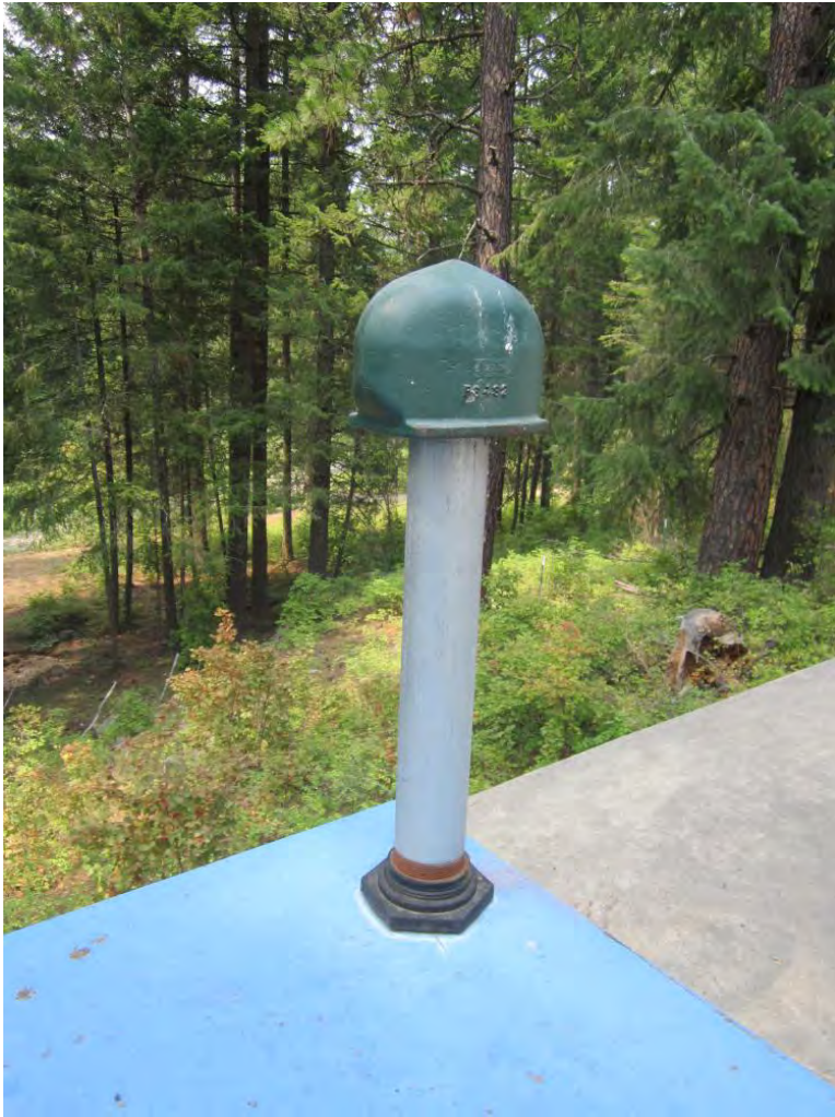
Photograph 87: Naples tank lid w screened vent
