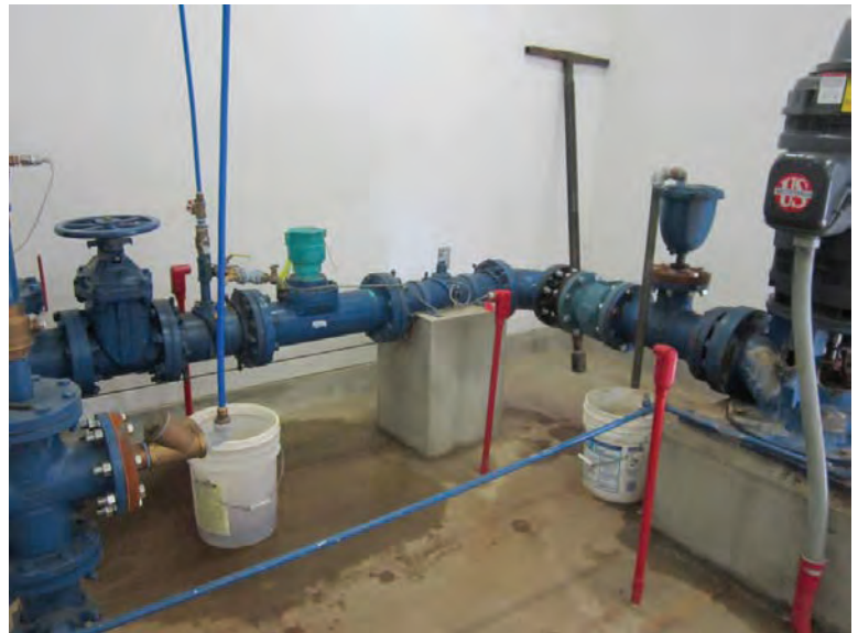
Photograph 32: Parker Canyon boosted discharge appurtenances
