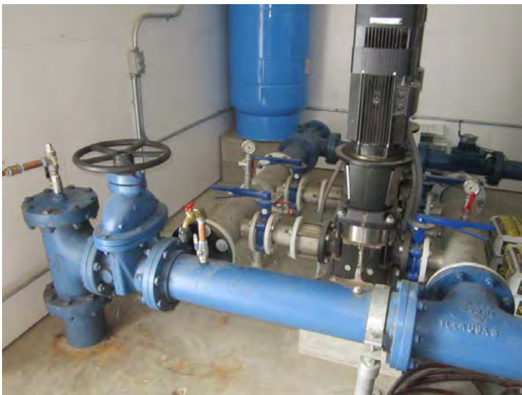
Photograph 39: Four Corners booster station
