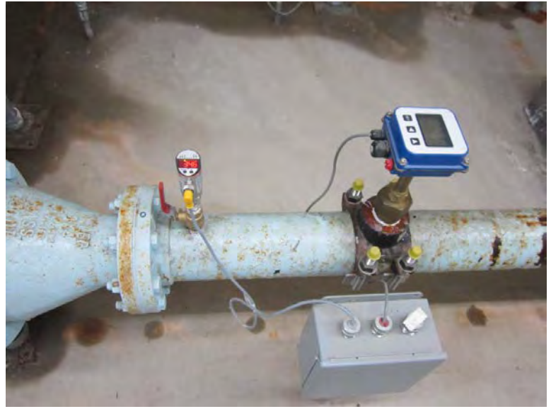
Photograph 62: Black Mountain boosted discharge flow meter
