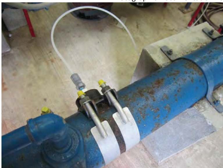
Photograph 13: Sodium hypochlorite injection quill
