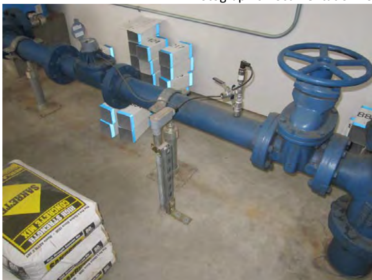
Photograph 45: Four Corners boosted discharge appurtenances
