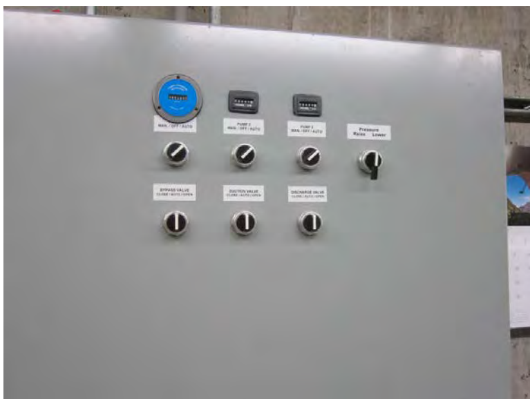
Photograph 67: Black Mountain booster pump controls
