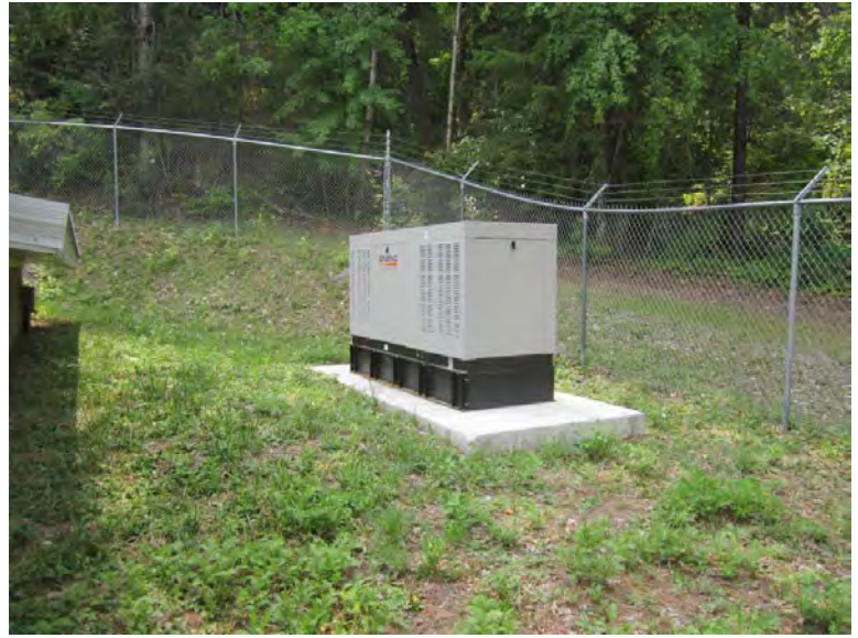
Photograph 58: Black Mountain booster station diesel generator
